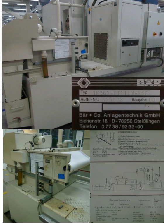
Periph. Rückpumpstat. (return pumping station)
